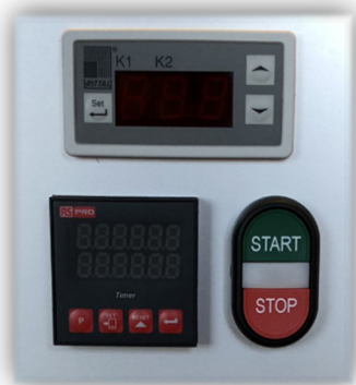
Control panel of warm-air blower
